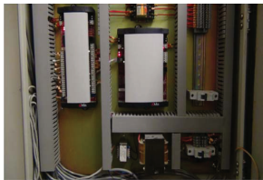
Fig. 22. Original wired MS/TP system
